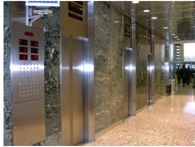
Turn off 1 of 4 elevators
