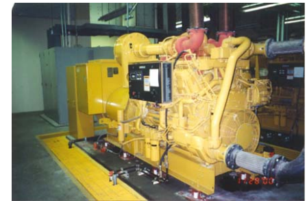
OR Turn on emergency generator
