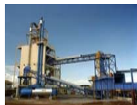
biomass power plant
