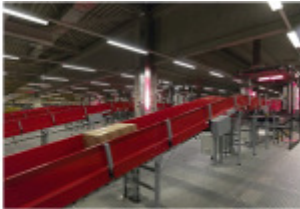
Warehouse - Ground to floor (with sorting machine)
